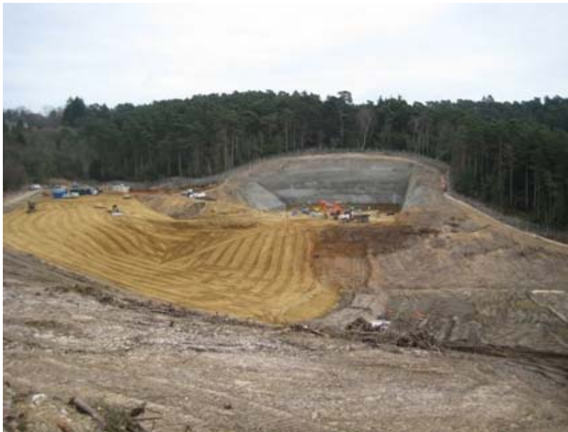
View of the south portal works for the A3 bypass and tunnel project March 2008 source HA website
